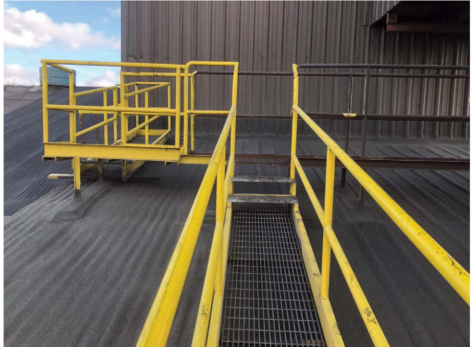
AN ACCESS WALKWAY AND ITS POSTS AND PENETRATIONS WERE SEALED WITH THE RE-COVER SYSTEM.
