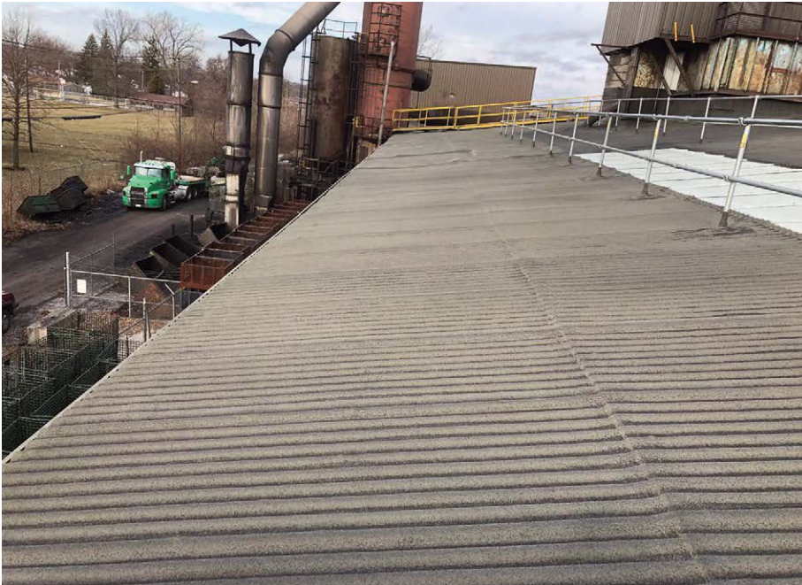
AFTER: FASTENERS AND LAP JOINTS ARE NO LONGER SUSCEPTIBLE TO WATER ENTRY WITH THE NEW MEMBRANE OF THE RE-COVER SYSTEM LAMINATED TO THE TRANSITE PANELS.
